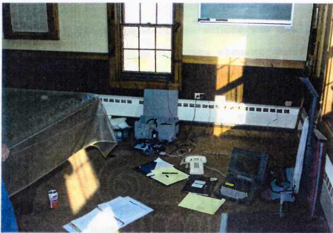
Fig. 2.7. View of the substation during the installation and testing of communications system
