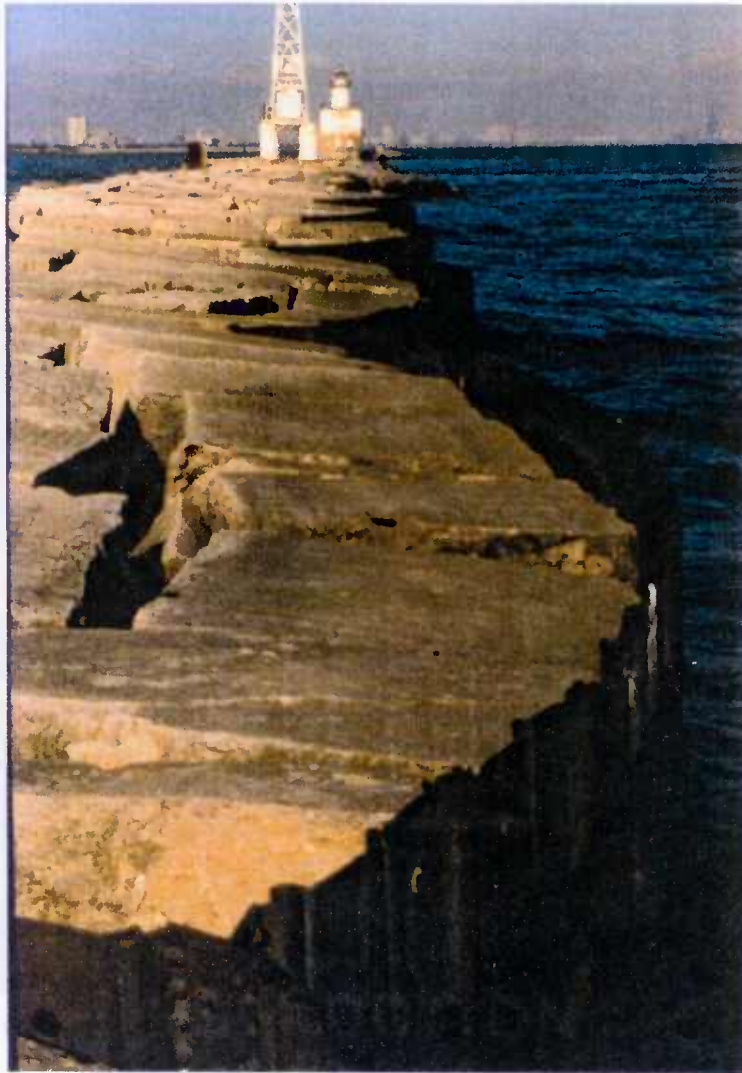
Fig. 1.7. View of the structure towards Southeast end indicating settled capstones
