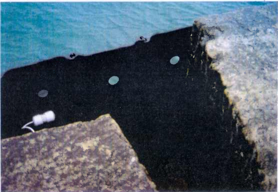
Fig. A.12. Protective PVC cover for the hoop strain gauge
