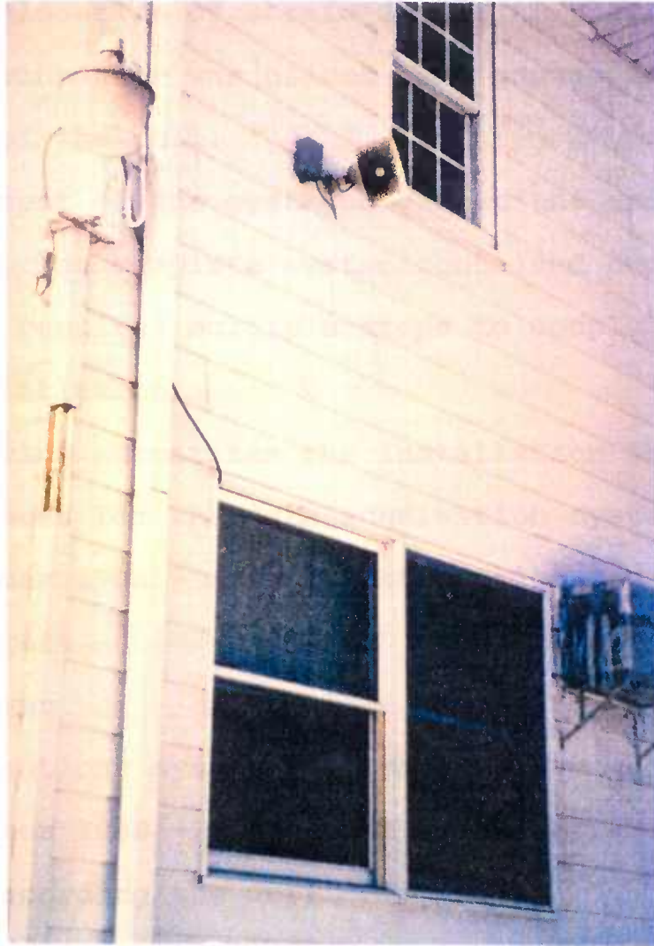
Fig. A.16 Installed communications antenna at the coast guard station
