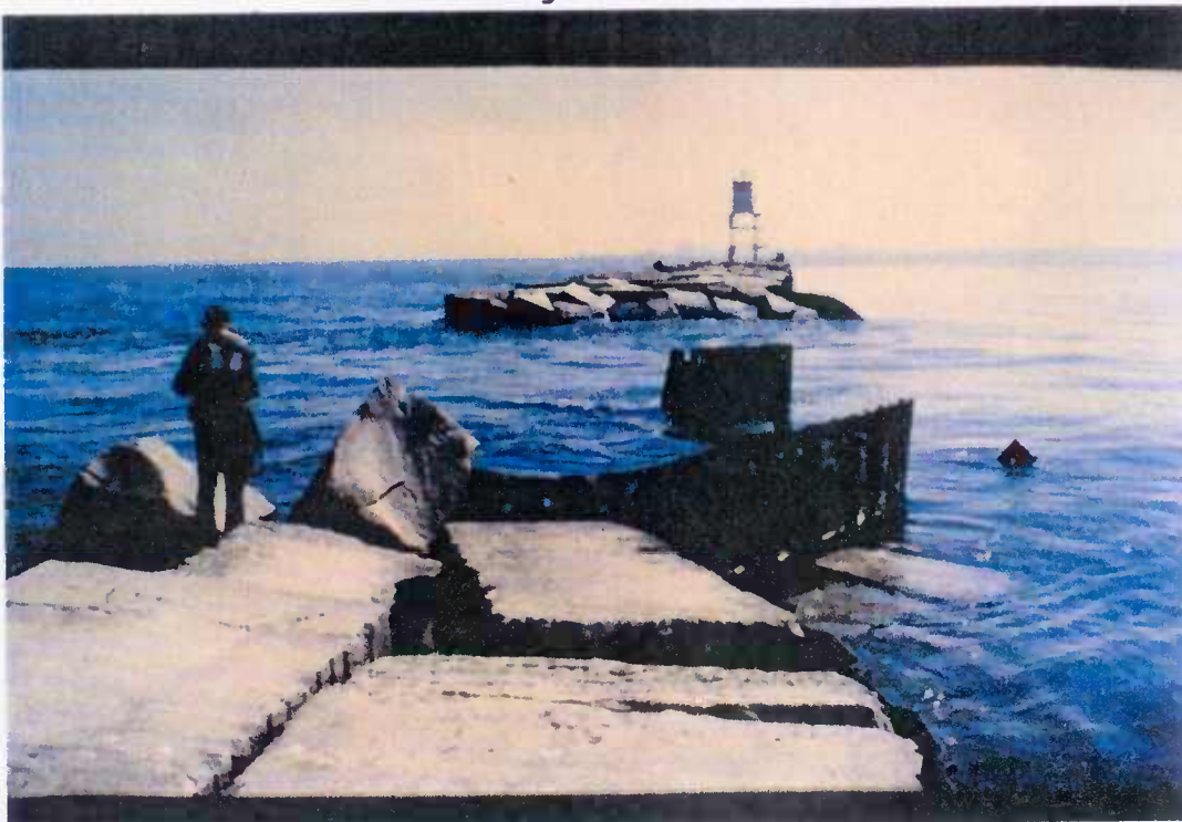
Fig. 1.4. View towards Southeast end of breakwater indicating failed cells
