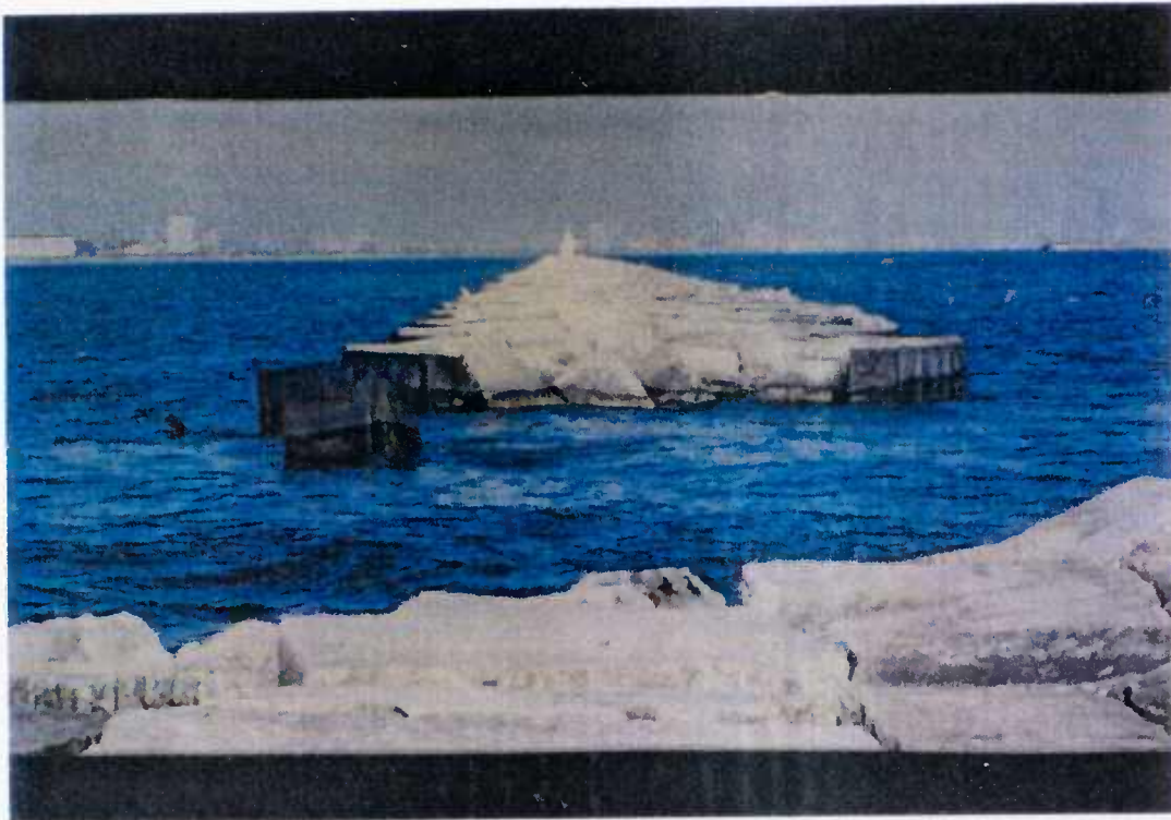
Fig. 1.3. View towards Northwest end of breakwater indicating failed cells
